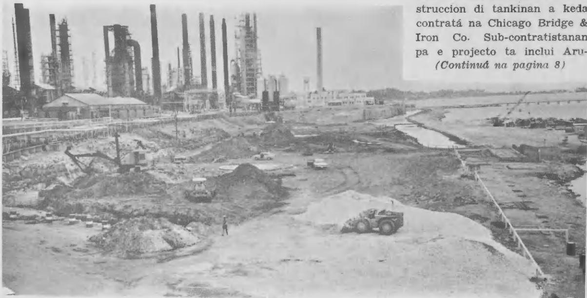
This site east of Powerhouse No. 1 is being prepared for erecting most of the units of Lago's Desulphurization Project. The site will be filled up with sand dredged from the lagoon. E sitio aki pariba di Powerhouse No. 1 ta ser prepara pa construi mayoria di e unidadnan di Lago su proyecto di Desulfurizacion. E sitio lo ser yena cu santo draga for di lagoen.
